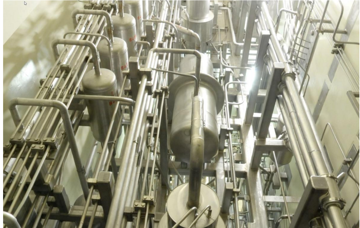
Vitrification Facility Karlsruhe
