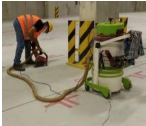
Figure 23. Process of crack enlargement at the ISF prior to being filled with resin
