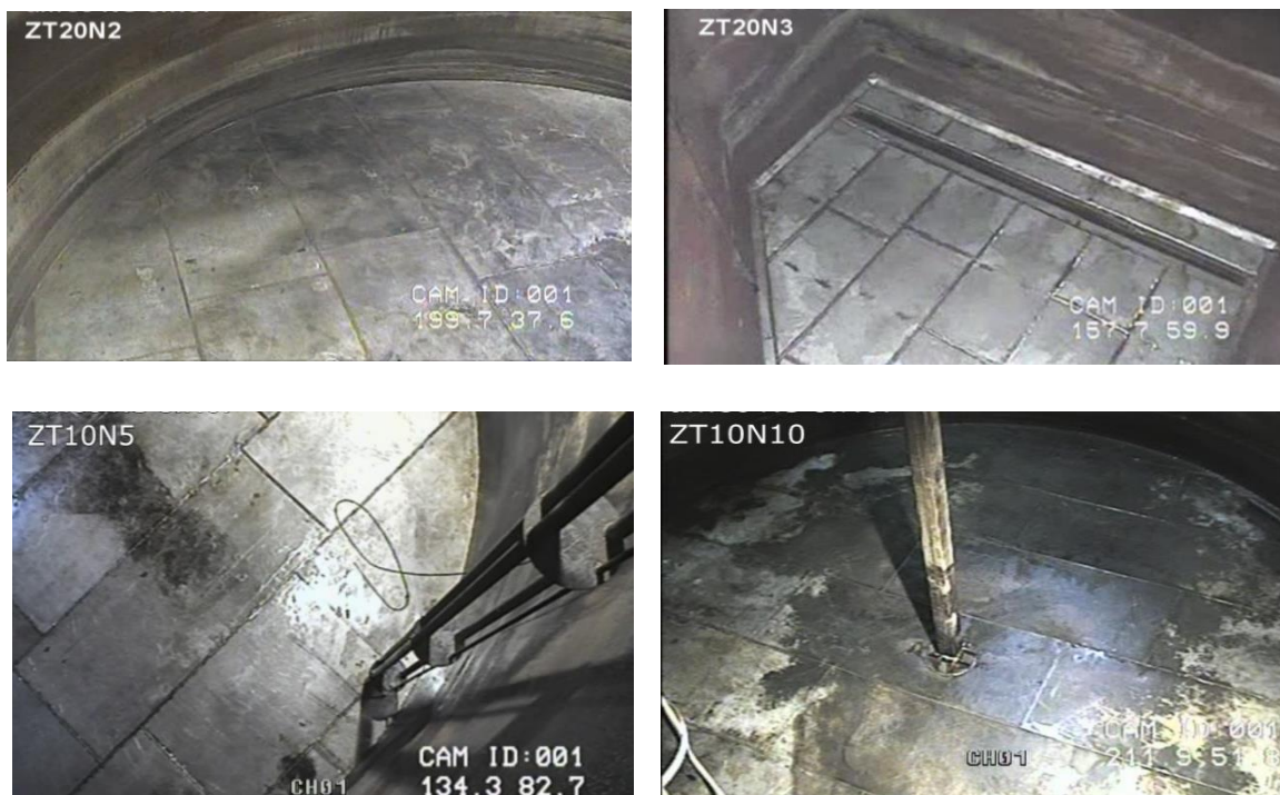
Figure 18. Cleaned storage tanks
