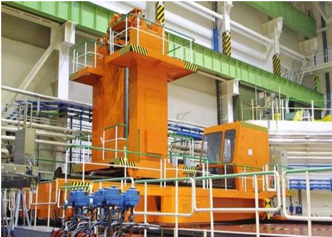
Figure 31. Equipment used to handle shielding assemblies over the spent fuel storage pool
