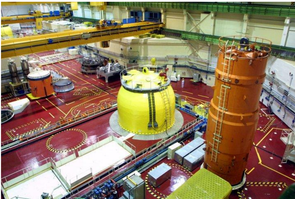
Figure 1: Reactor Hall at Bohunice V1
