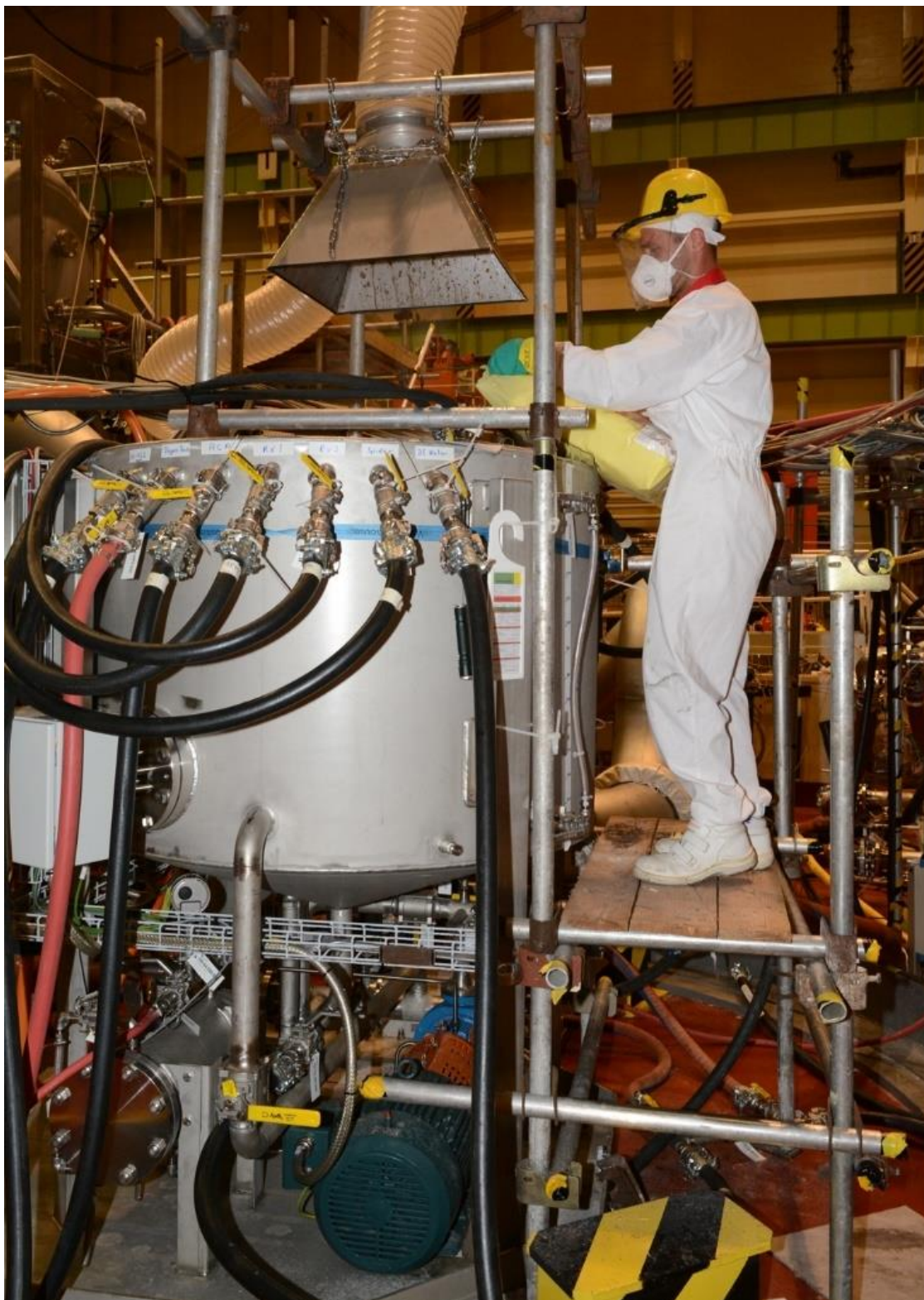
Figure 6: Chemical dosing into the Venting/Mixing Tank.
